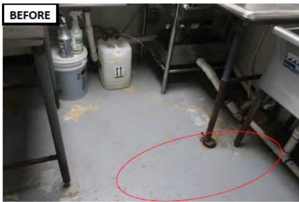
Photograph 7: Prep kitchen floor (9/23/2022).
