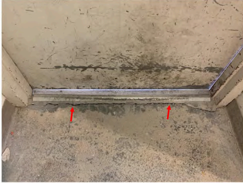
Photograph 6: Ground-level slab at stair exterior door at west elevation.
