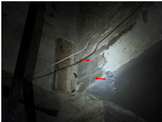
Photograph 9: Cracking to south face of beam 2RSB-7.
