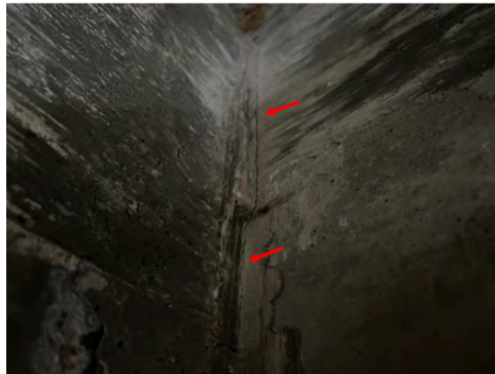
Photograph 17: Vertical crack between beams 2RSB-7 and 2RSB-3.
