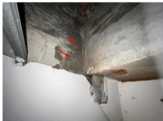
Photograph 11: Beam-column joint overview. Diagonal crack to north face of 2RSB-7.
