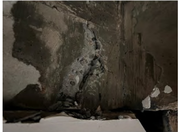
Photograph 13: Diagonal crack in Photograph 12 continues into beam.
