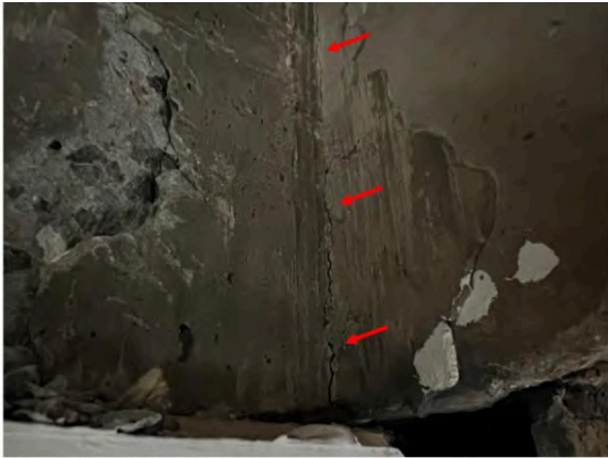
Photograph 16: Vertical crack between beams 2RSB-7 and 2RSB-3.
