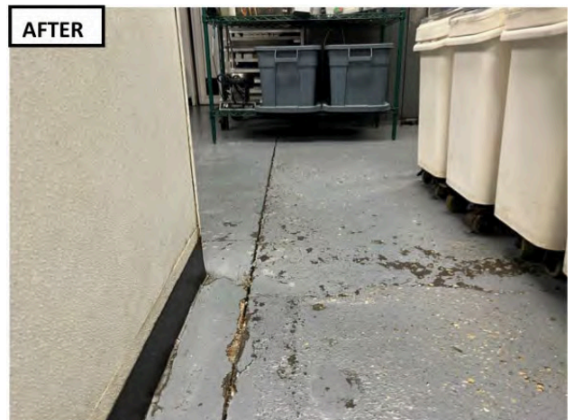
Photograph 12: Joint in kitchen floor (11/28/22).
