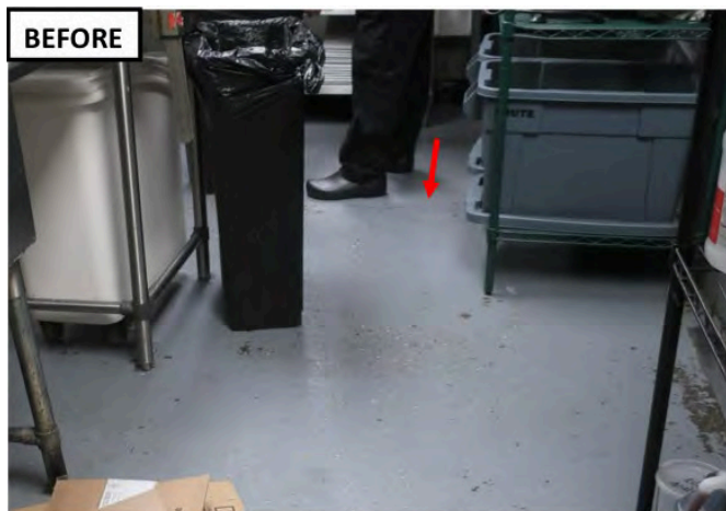
Photograph 11: Joint in kitchen floor (9/23/22).
