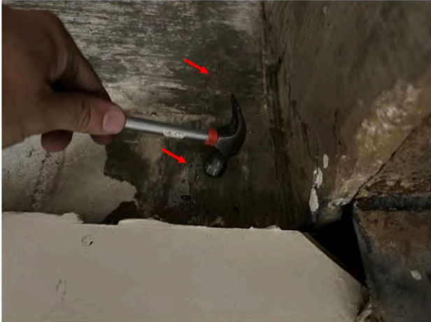
Photograph 12: Close-up view of crack shown in Photograph 11. Delaminated concrete chipped off.
