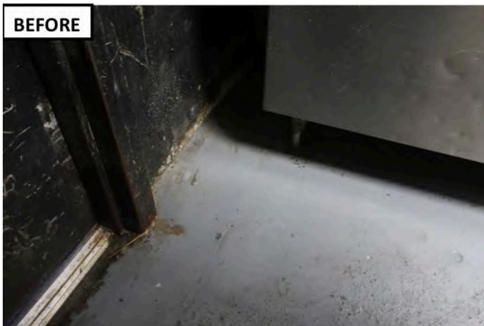
Photograph 15: Floor adjacent to double-doors (9/23/22).
