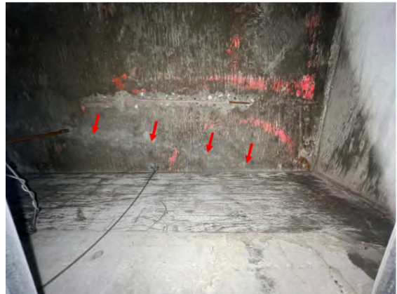
Photograph 18: Diagonal crack on underside of second-story floor slab adjacent to beam 2RSB-7.
