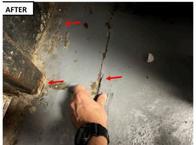
Photograph 16: Floor adjacent to double-doors (11/28/22).
