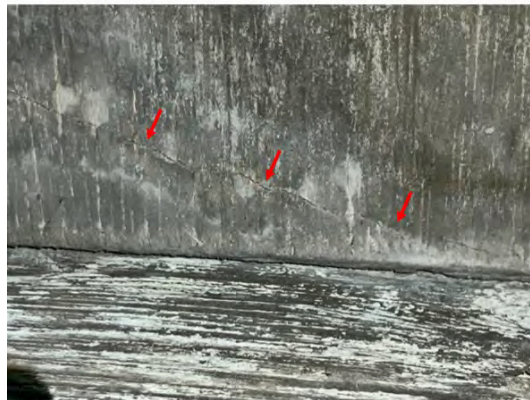
Photograph 19: Close-up view of the crack in Photograph 18.
