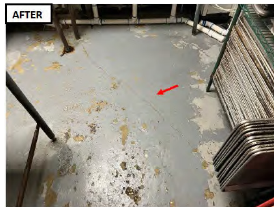
Photograph 8: Prep kitchen floor (11/28/2022).
